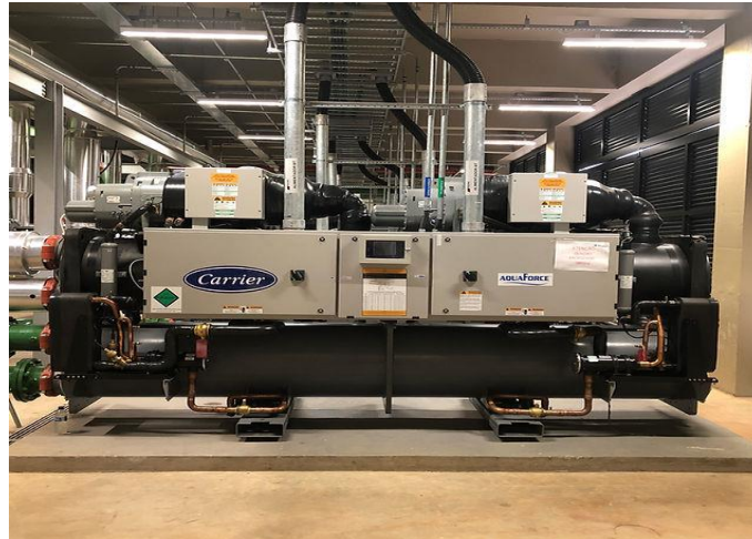
Figure 3: Chilled Water Center.
